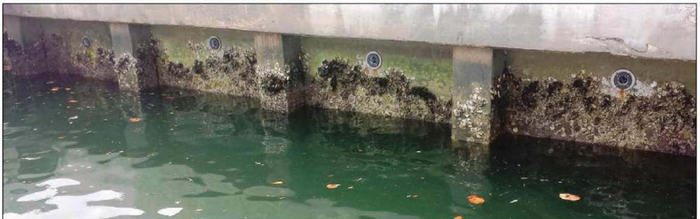
Lake Park Marina in Lake Park, Florida (not shown here), renovated its failing seawall with 150 weep holes from JET Filter. The weep holes relieve hydrostatic pressure behind the wall, providing a mechanism for water to drain through the seawall.
